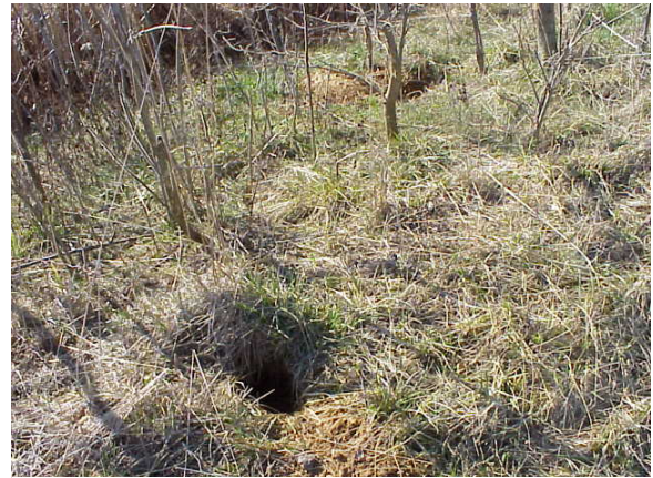
Figure 1.20: Animal burrow in pond embankment.
