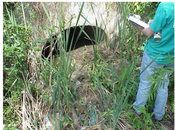
Figure 5.11: Excessive vegetation near an outfall
