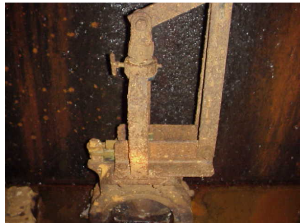
Figure 1.19: Corroded plumbing and valve.
