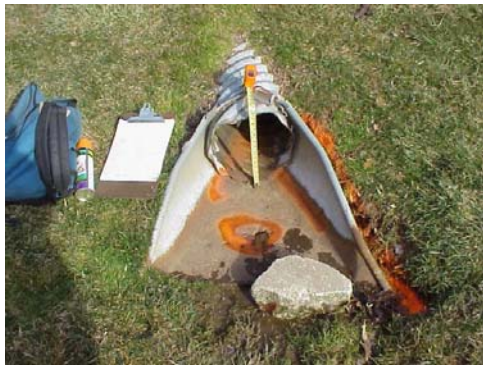
Figure 4.1: Marking outfall deficiencies.
