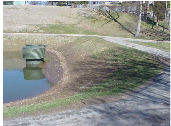
Figure 5.10: Bare soils on embankment and slopes
