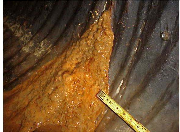
Figure 5.6: Soil entering open pipe joint.
