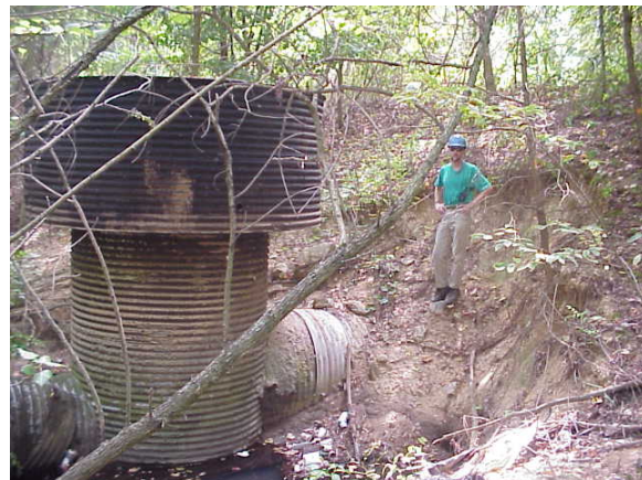
Figure 1.8: Severe erosion around riser and barrel
