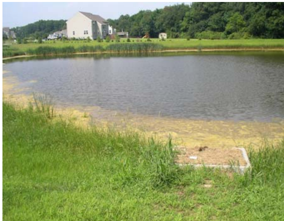
Figure 1.5: Flattop riser covered with debris.
