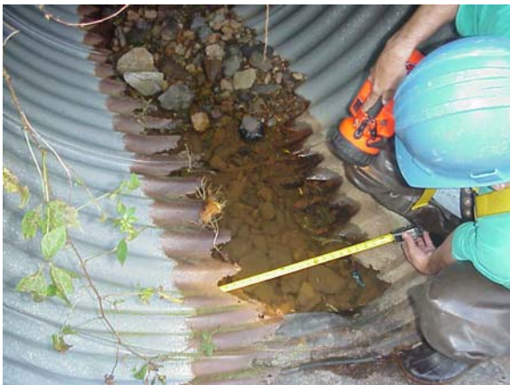
Figure 1.7: Pipe invert abrasion
