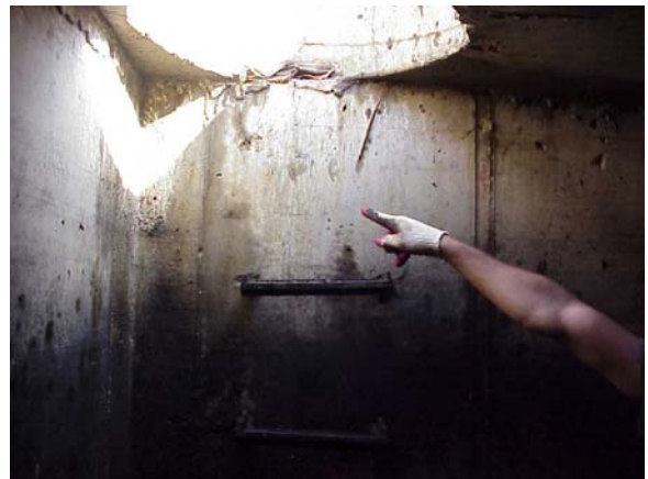
Figure 5.21: Missing manhole step
