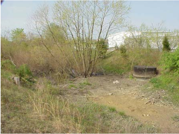
Figure 1.13: Sediment accumulation in a dry pond
