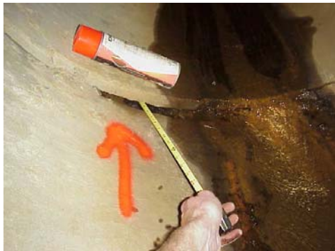
Figure 4.3: Marking pipe joint separation
