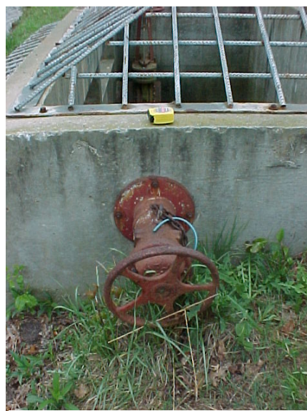
Figure 5.25: Valve outside riser.
