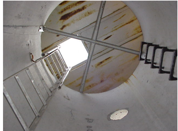
Figure 1.16: Ladder and steps in riser.
