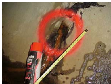
Figure 5.8: Rust intrusion demonstrates improper pipe joint.
