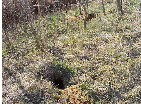
Figure 5.27: Animal burrow in pond embankment.
